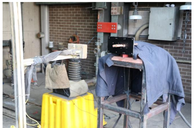
Figure 2 View of the horizontal parallel electrodes, no box
